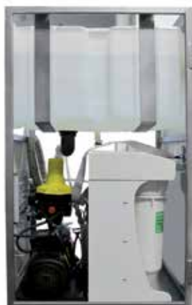
Water tank and pressure boosting system side view
