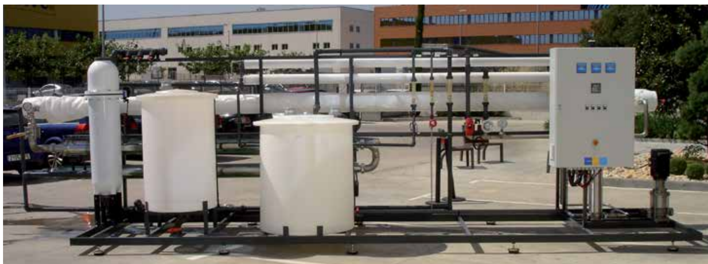
Double pass RO plant for the production of high quality water for car wash.
