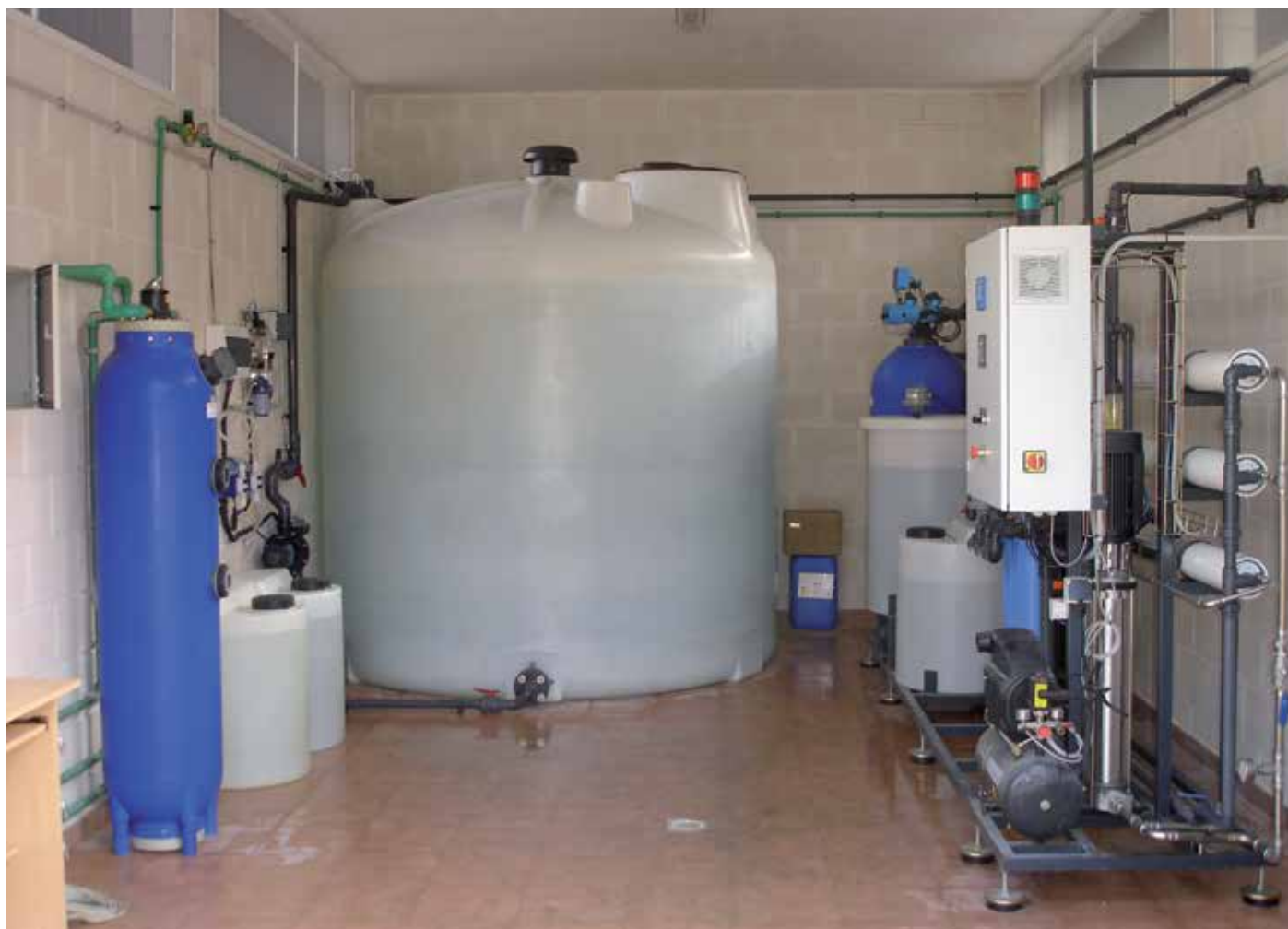
Double pass RO plant to supply drinking water to a small Mediterranean village.
